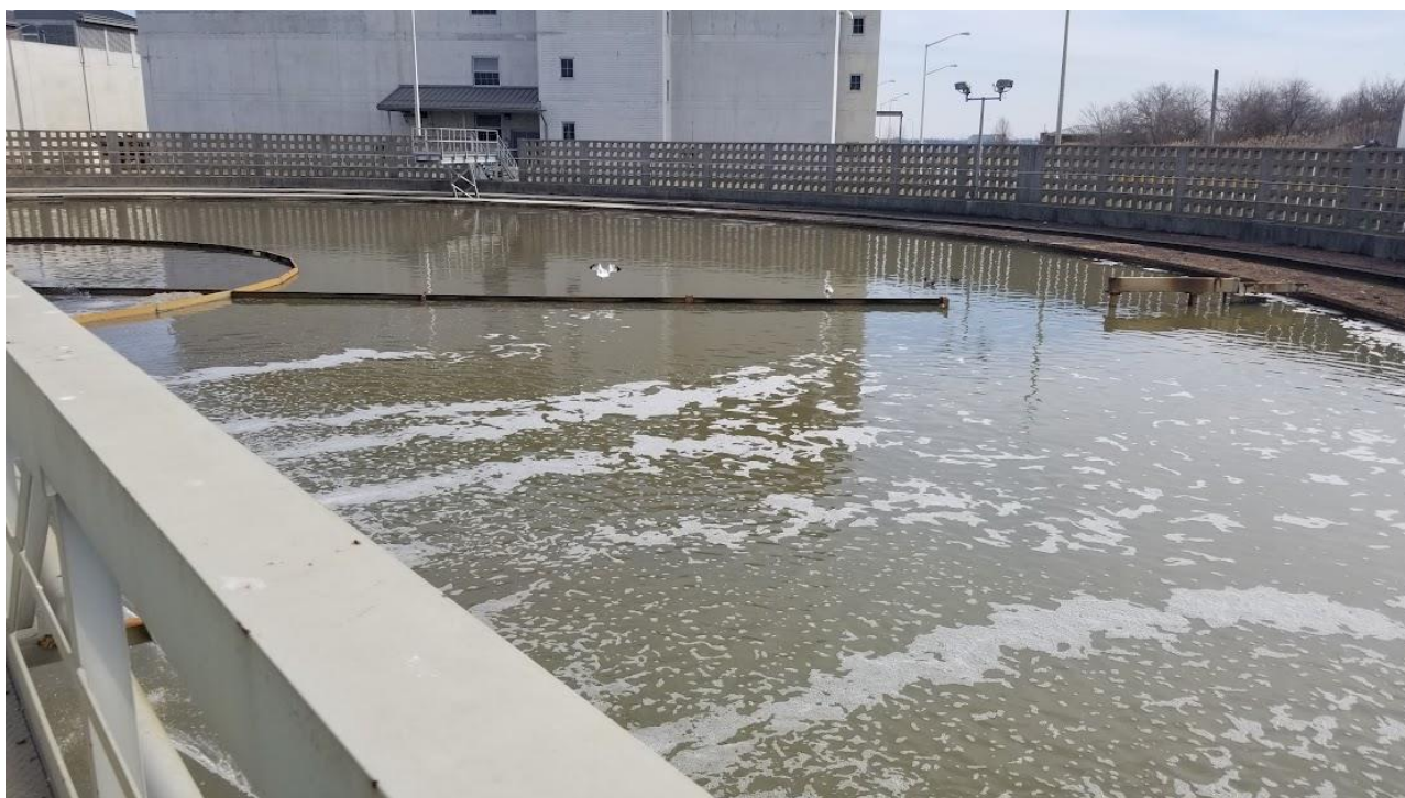
Figure 5a: Scrapper arm in Clarifier #4 is missing.
