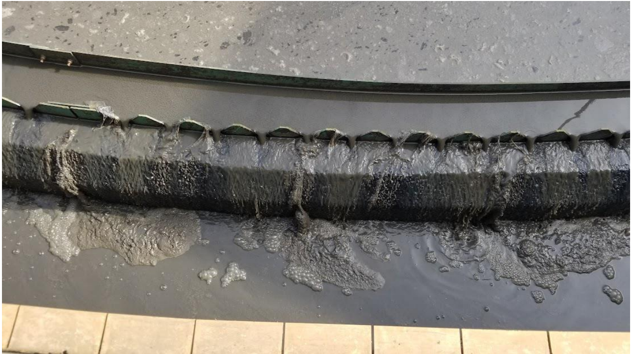
Figure 2c: Close up view of the sludge that have previously been spilled out of the V- notch weir within GST #1.
