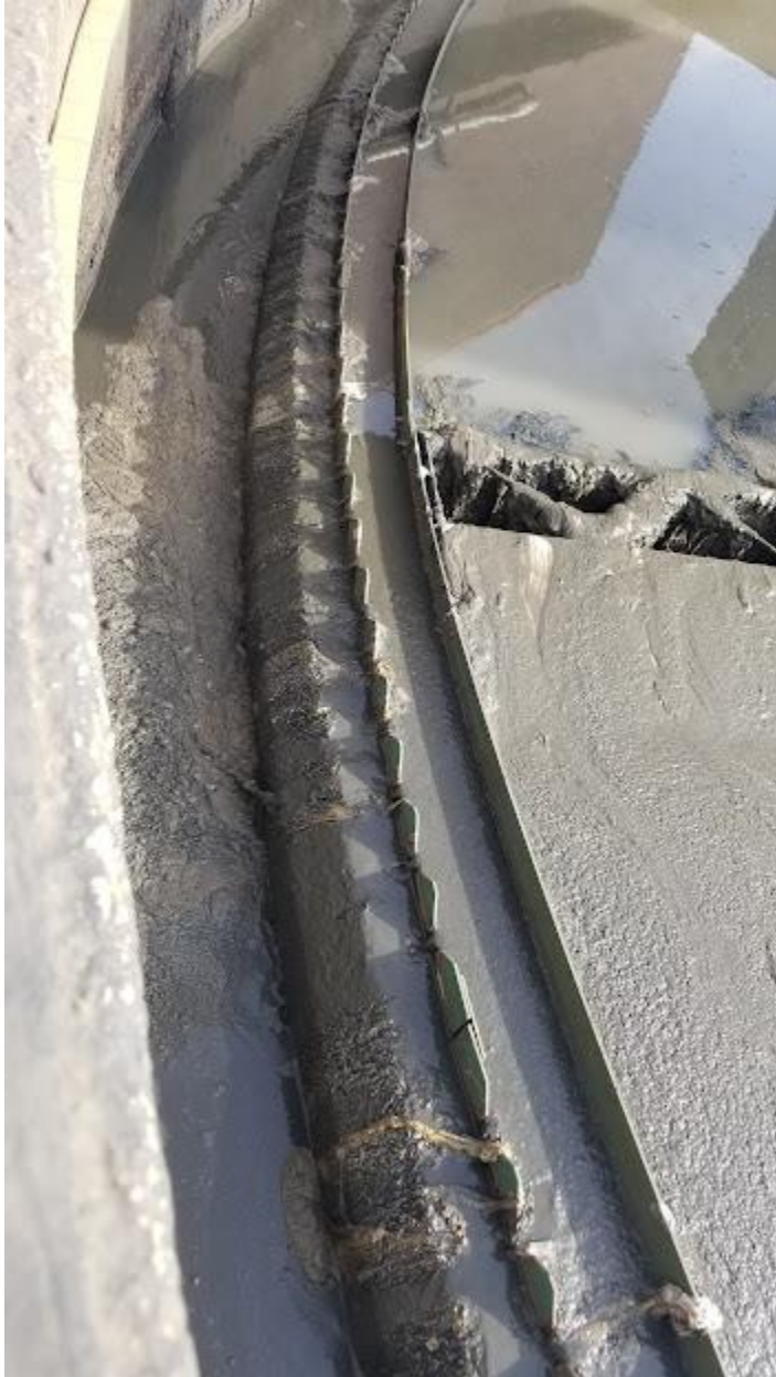
Figure 2e: Sludge that have previously been spilled out of the V- notch weir within GST #2.
