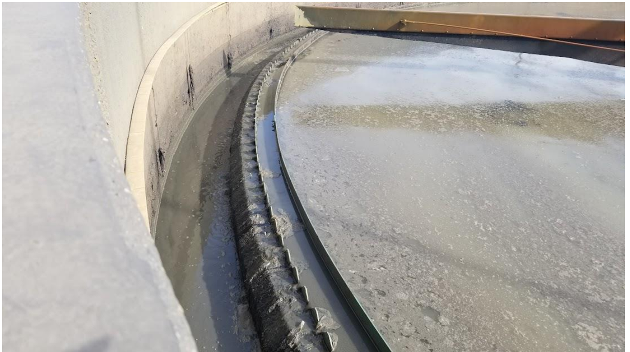
Figure 2b: Sludge next to the outer side of the weir within GST #1. Rags next to the V-notch weir. Scrapper arm is above the water surface level.
