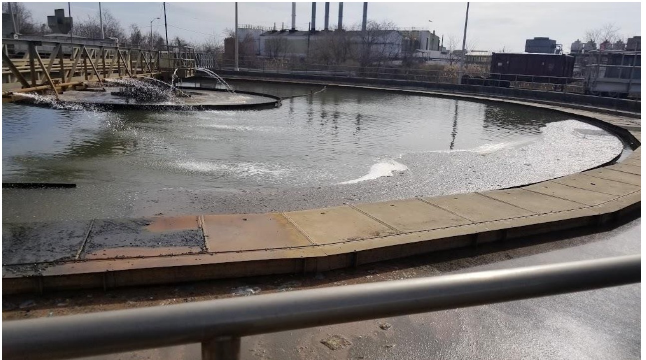
Figure 5e: Scum accumulation within Clarifier # 5b.
