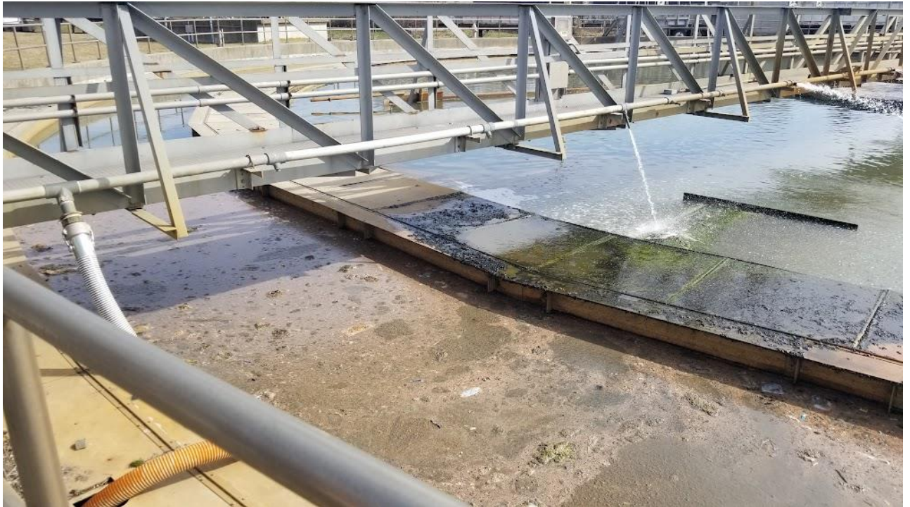
Figure 5d: Scum accumulation within Clarifier #5b.
