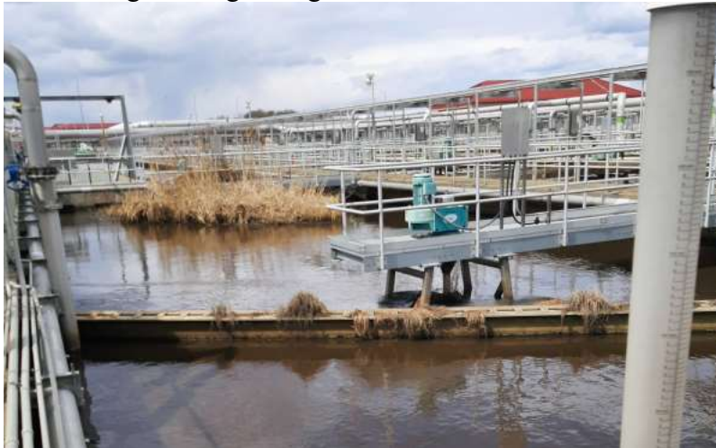
Vegetation growing in the reactor 3/26/22
