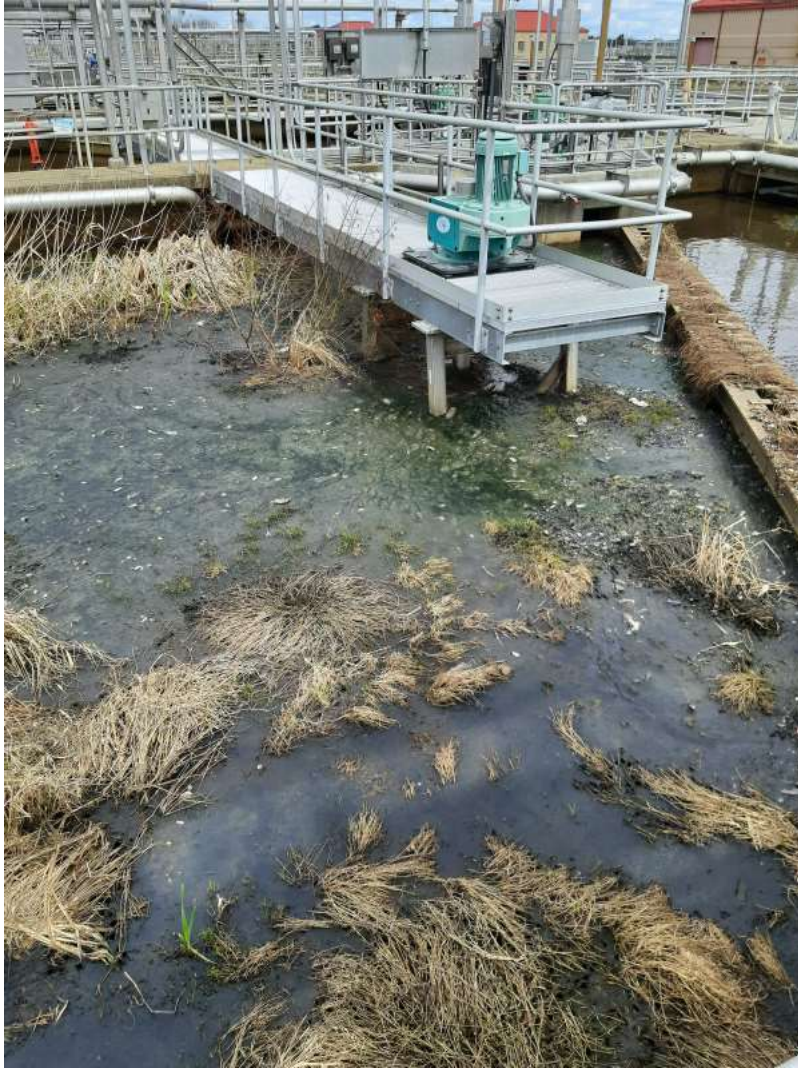
Mixer unable to turn properly due to solids in the reactor 3/26/22
