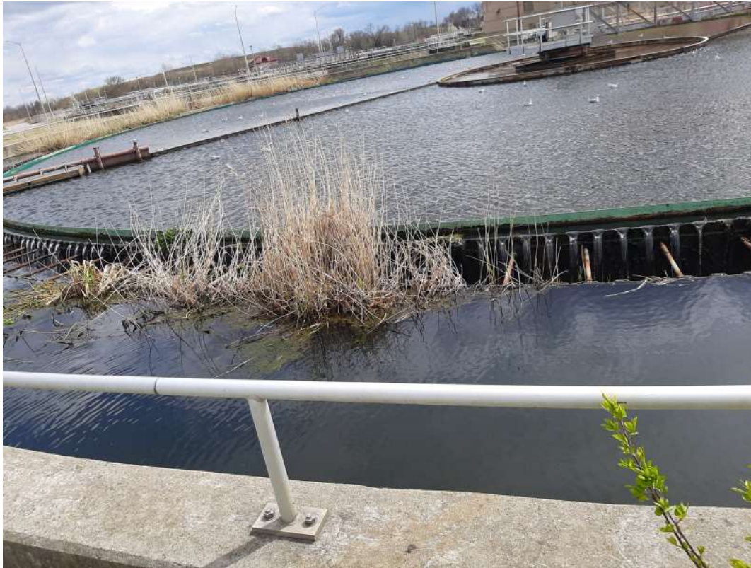
3/26/22 Secondary clarifier- vegetation and solids clogging the system and short-circuiting of the weirs.
