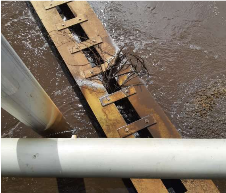
3/26/22 vegetation growing in reactor
