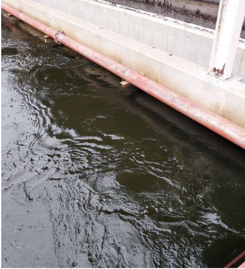
Effluent from the DN filters going to the sand filters. 3/26/22
