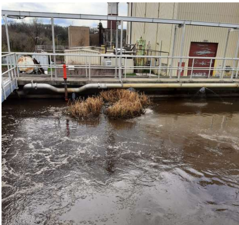
3/26/22 Vegetation growing in solids accumulated in one of the reactors
