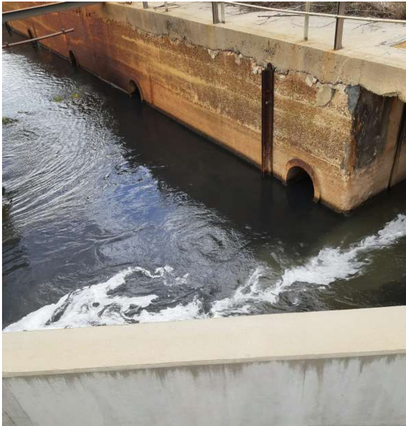
Turbid dark grey wastewater flowing from the PST primary treatment to the biological reactors 3/26/22
