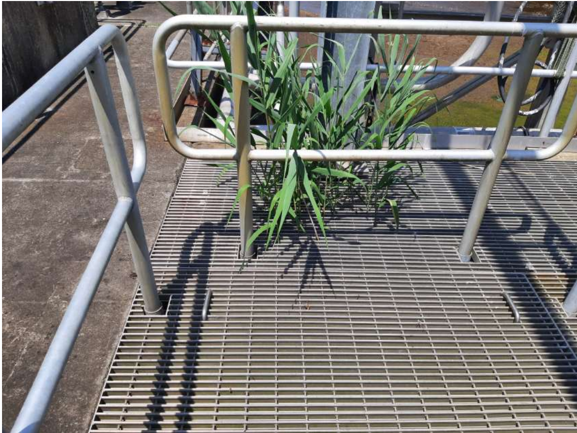
6/2/22 Reed grass coming up through grating above a reactor basin.
