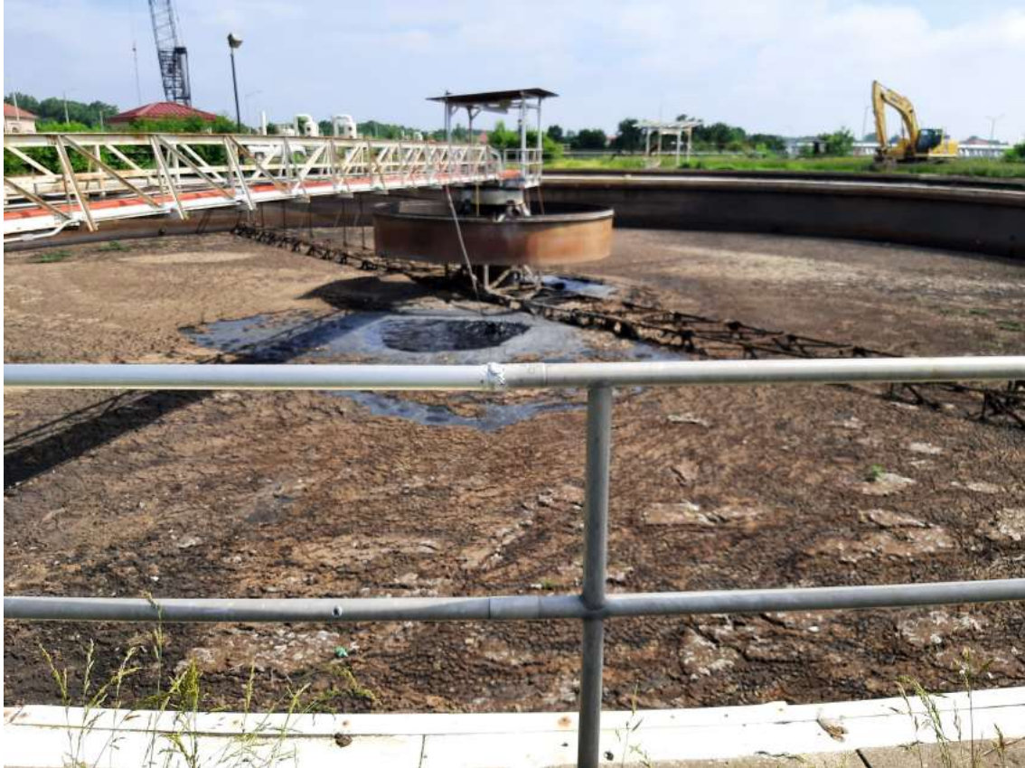
6/2/22 Nonfunctioning PST #1 being drained
