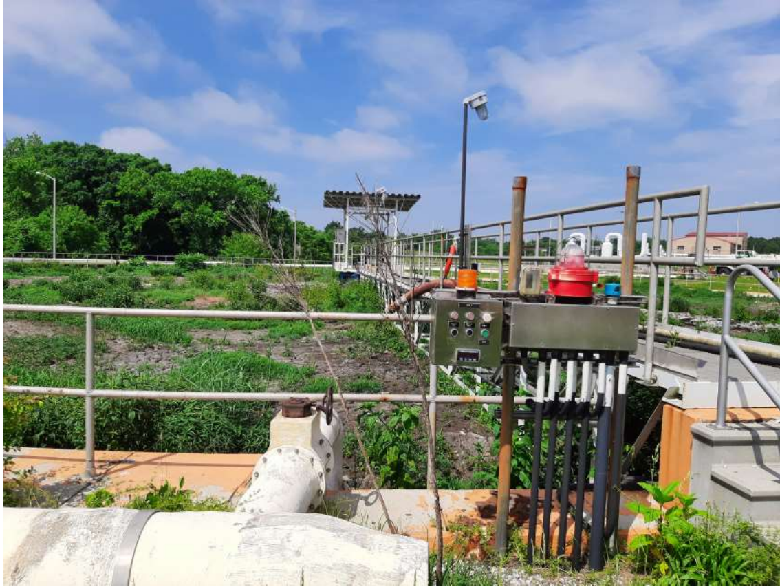
6/2/22 PST #5 Nonfunctioning PST filled with vegetation
