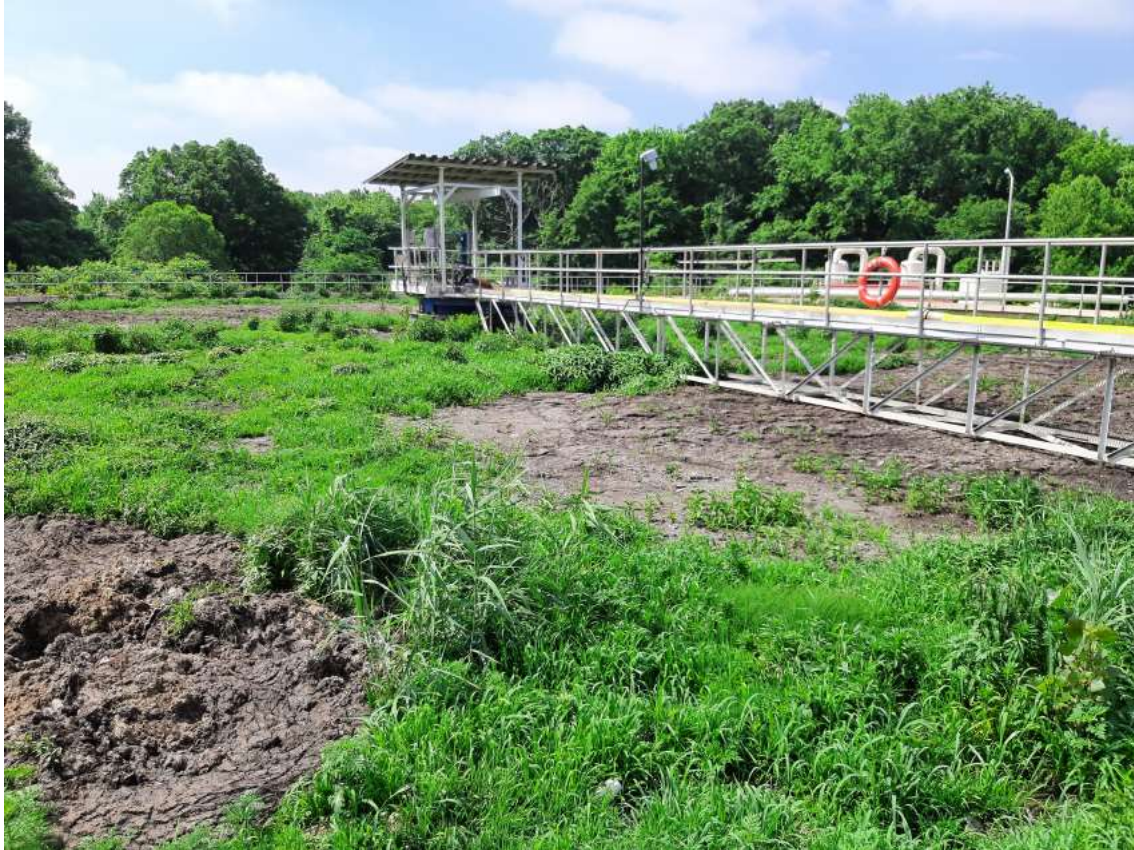
6/2/22 PST #6 Nonfunctioning PST filled with solids and vegetation
