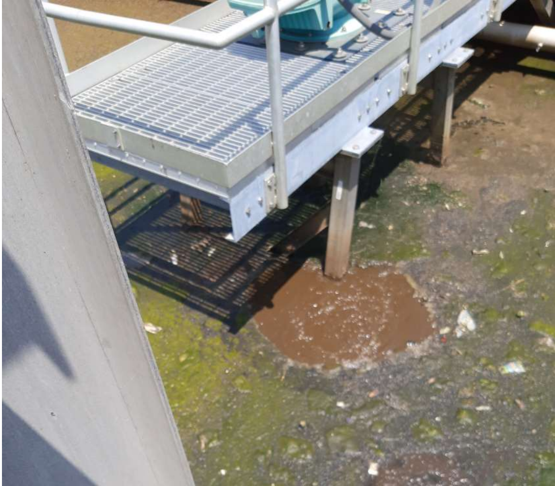
6/2/22 Mixer in reactor barely turning. Note accumulation of solids due to poorly functioning equipment.
