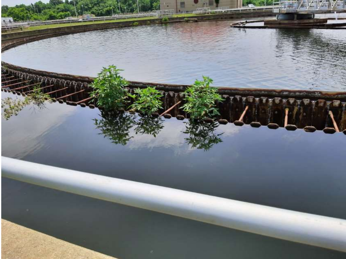
6/2/22 Vegetation growing in secondary clarifier 14A
