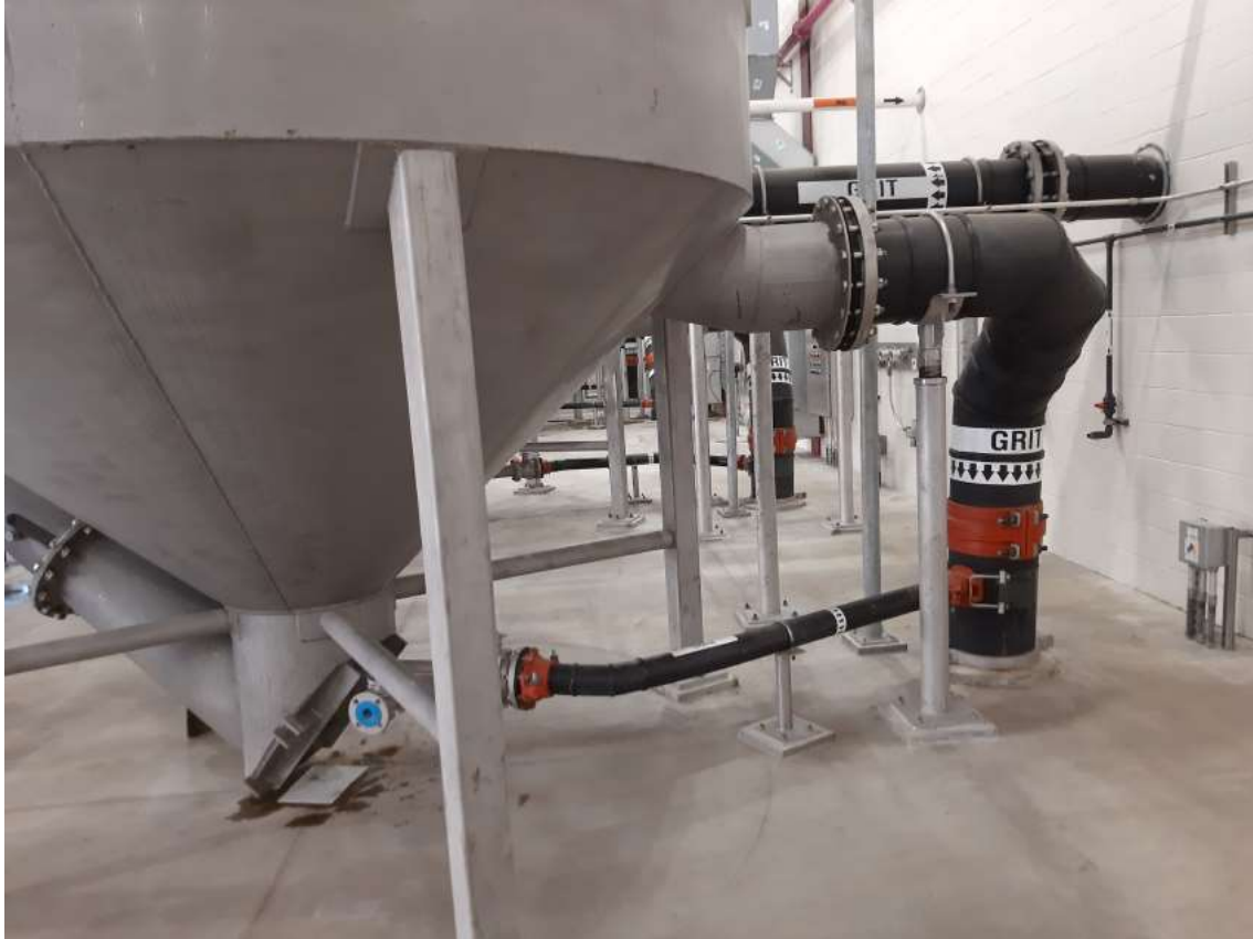
6/2/22 Grit dewatering system
