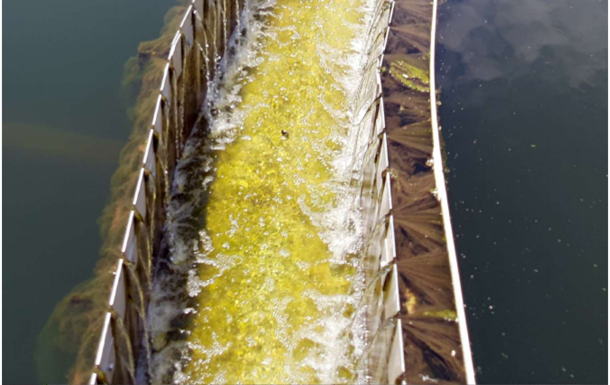
6/2/22 Clarifier # 17B algae growing on the weirs
