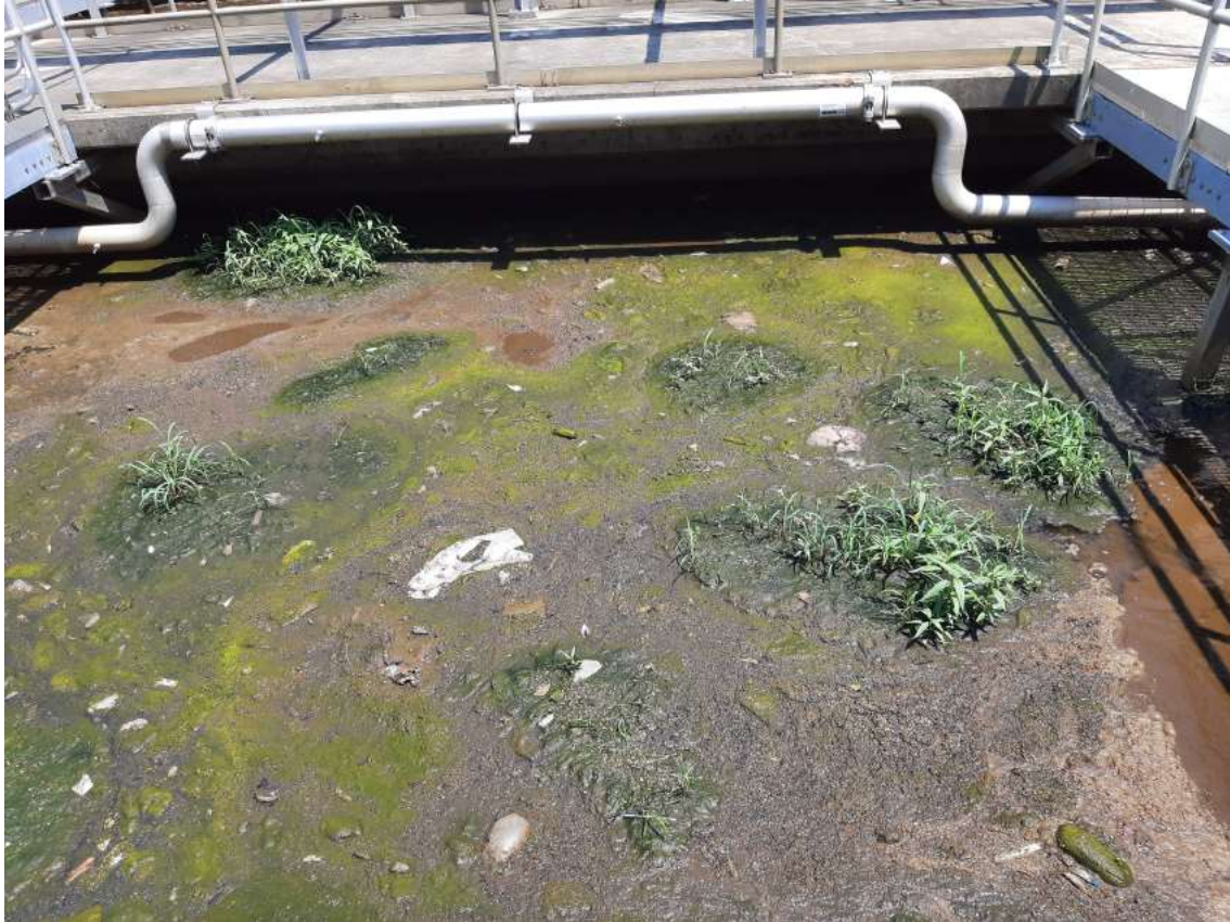
6/2/22 Heavy layer of solids and vegetation preventing proper operation of the reactor
