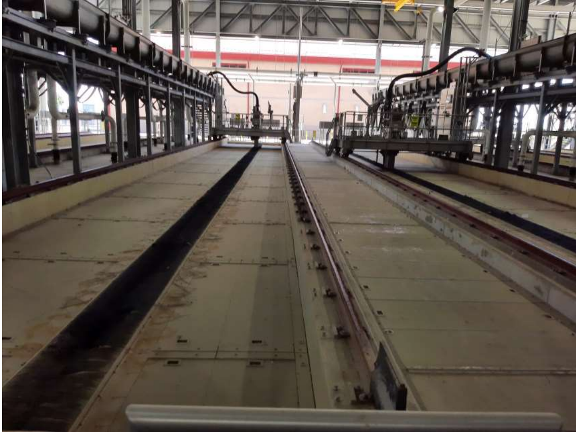
6/2/22 Grit removal system- Traveling Bridges suction the grit from the tanks to overhead conveyors that convey the grit to a dewatering system consisting of spinning classifiers.
