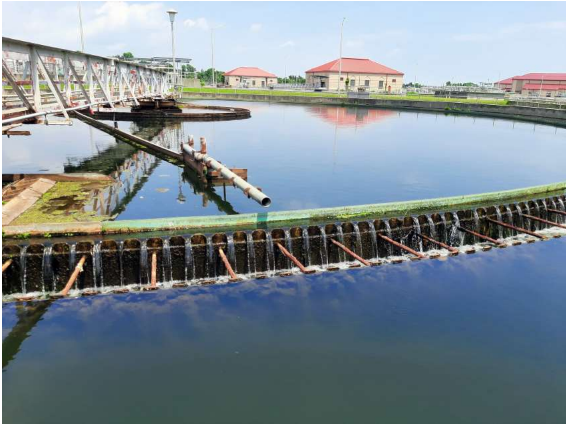
6/2/22 Secondary clarifier 16 B missing scraper flange.
