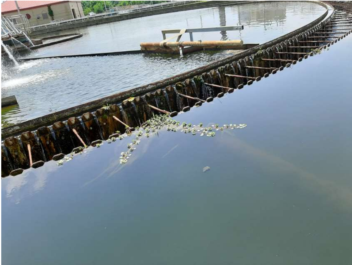
6/2/22 Vegetation growing in a secondary clarifier
