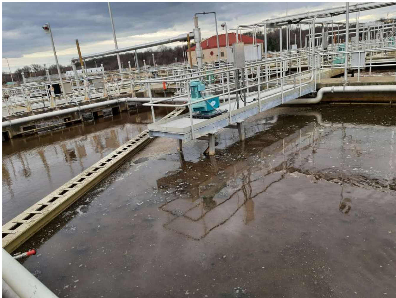
1/26/23 Activated Sludge Plant #3. Mixer problems in this reactor.
