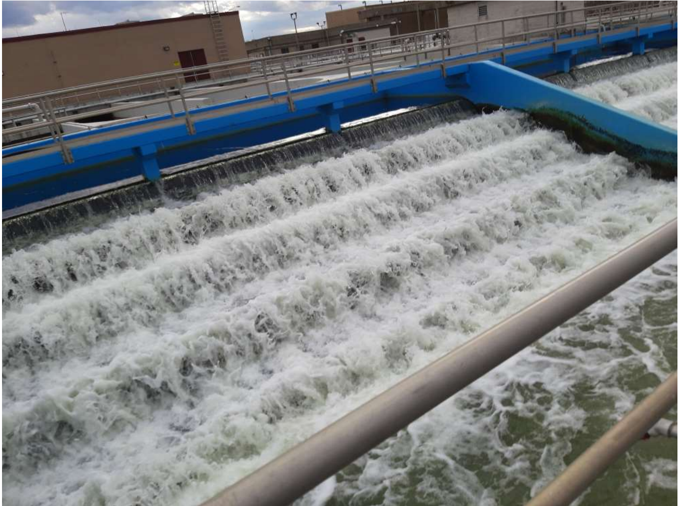
1/26/23 Final Effluent at the step aeration system
