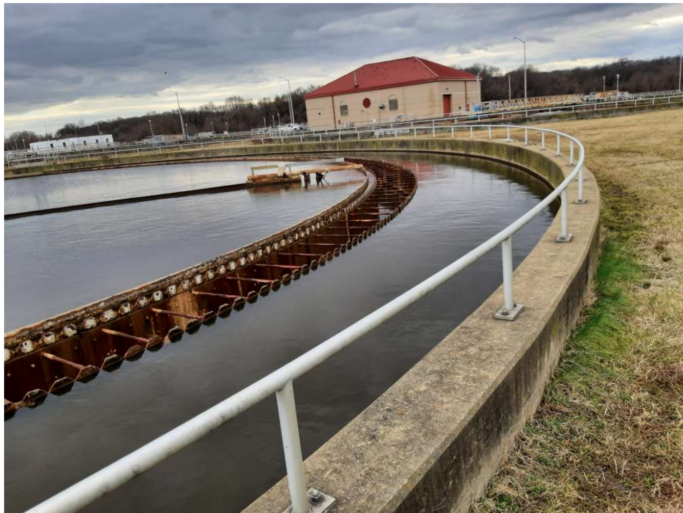
1/26/23 Secondary clarifier 14A – Missing skimmer flap.
