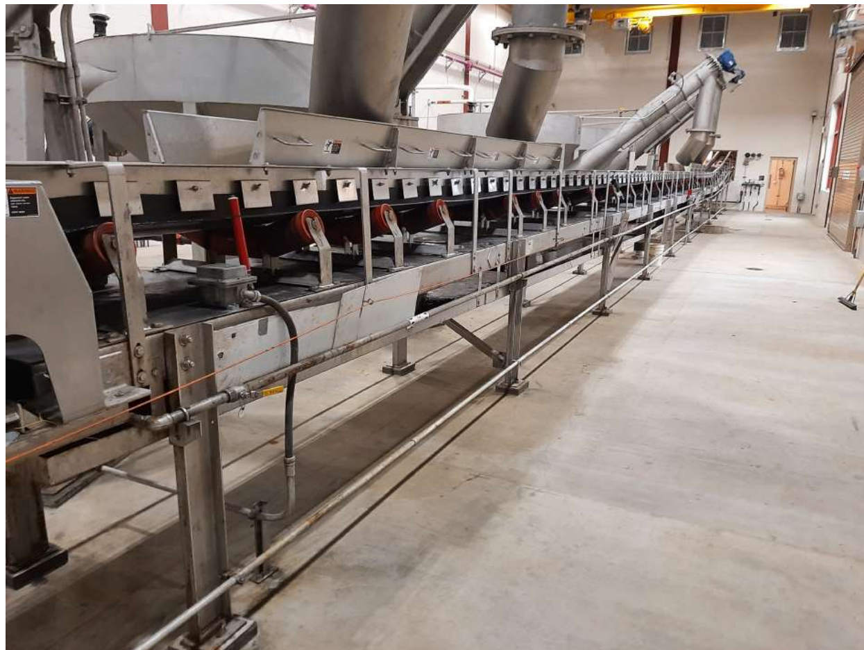
1/26/23 Grit removal area
