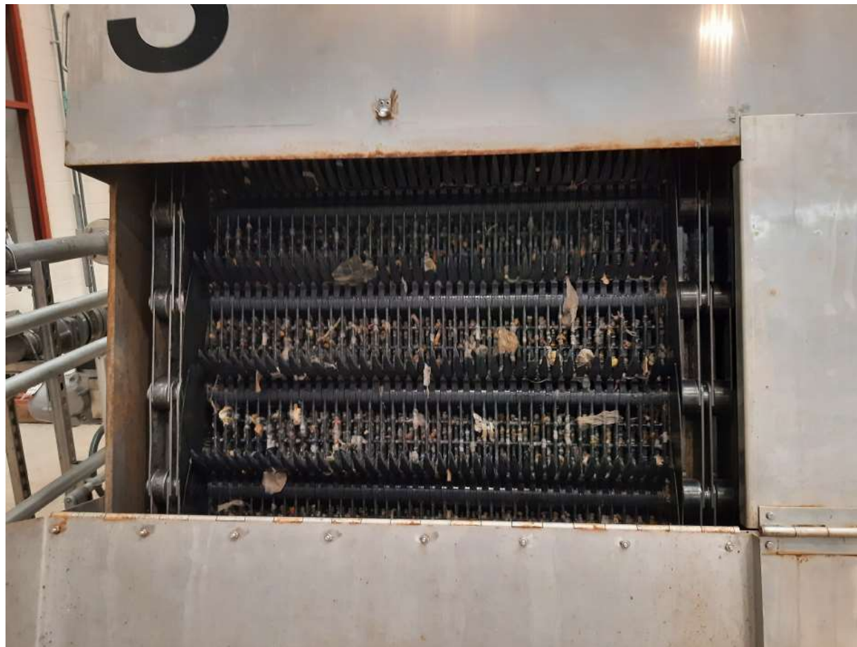
1/26/23 Fine screening unit in service.
