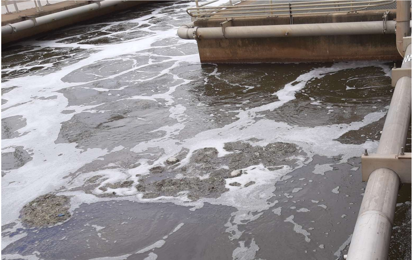
1/26/23 Reactor in the Activated Sludge Plant #3.
