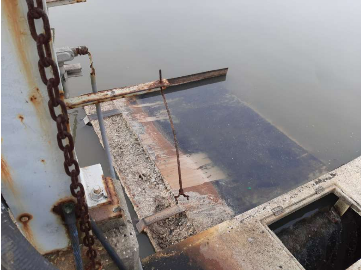
Picture of PST #8's clogged scum trough during 12/14/22 inspection. Clogged scum troughs are a persistent problem.
