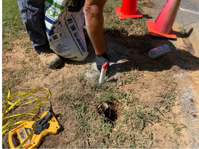
Photograph: 4 Description: View of A-Zone constructing temporary well at SB-4 location. HRSC OIP borehole visible next to temporary well.
