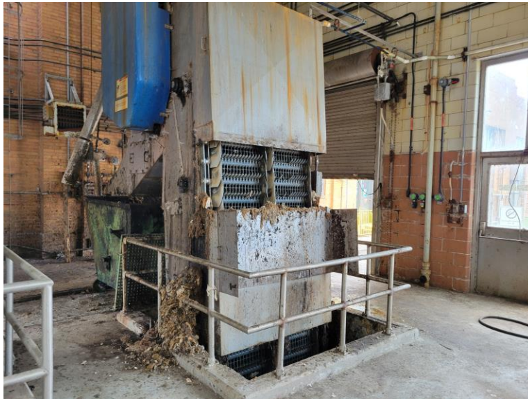
Image 1: IPI Building, Bar Screen #2.
