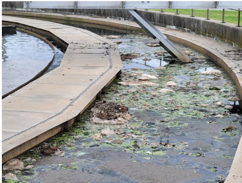
Image 9: Debris observed in Clarifier #5b.
