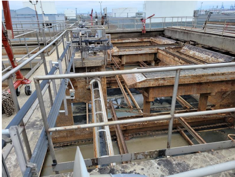
Image 6: PST #1, new troughs and actuators installed.
