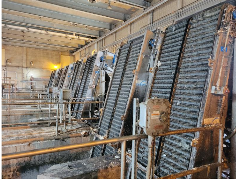
Image 2: Fine Screen Facility.
