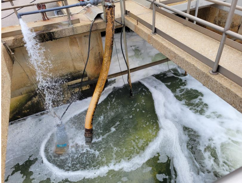
Image 11: Final Effluent from Chlorine Contact Chambers.
