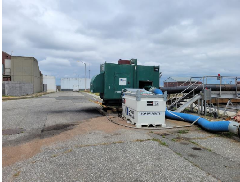
Image 7: Temporary United Rental Pump, adsorbent material.
