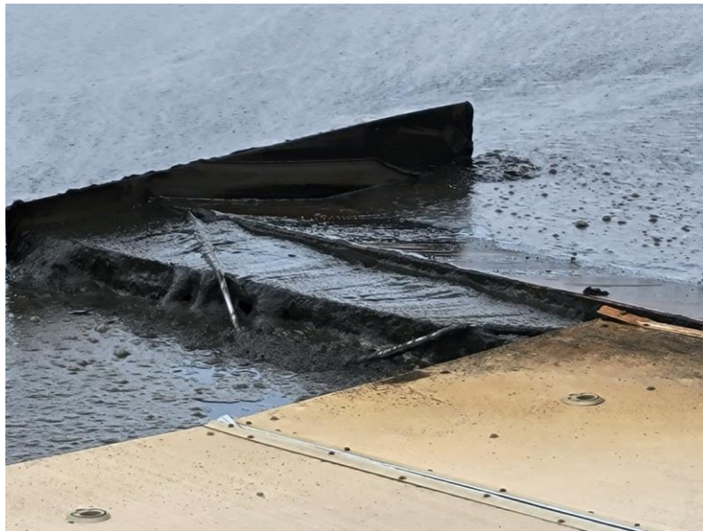
Image 8: Secondary Clarifier #1, clogged scum trough.
