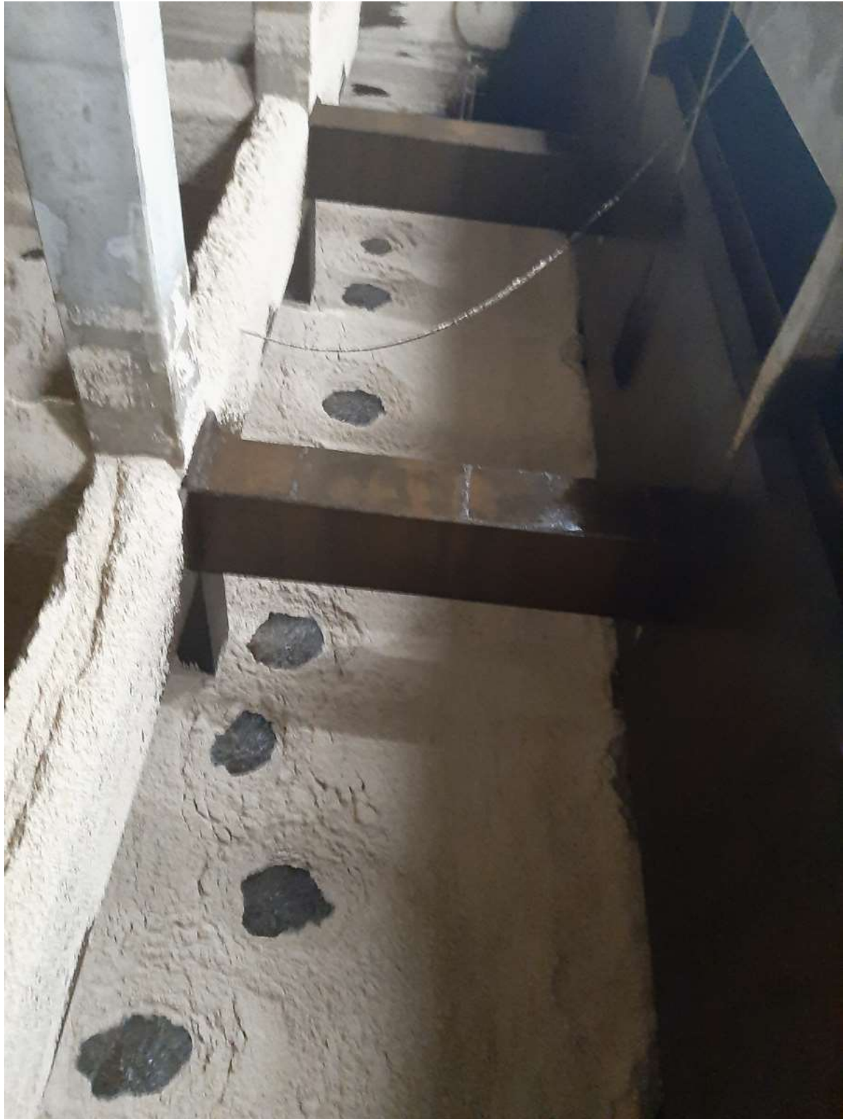
Picture taken 11/2/22 of backwash mud well showing media accumulation.
