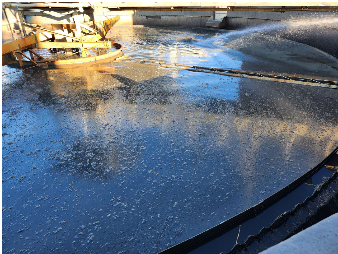
1/30/23 GST#1 scum layer on the surface due to inability of the skimmer arm to function. Scum and trash observed on the weirs.
