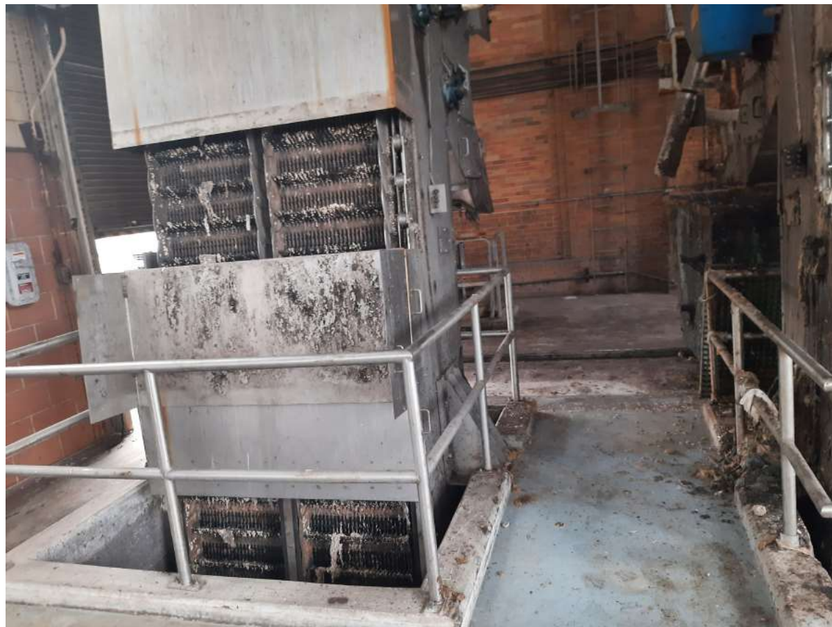
1/30/23 One of the screening units at the industrial influent screening facility
