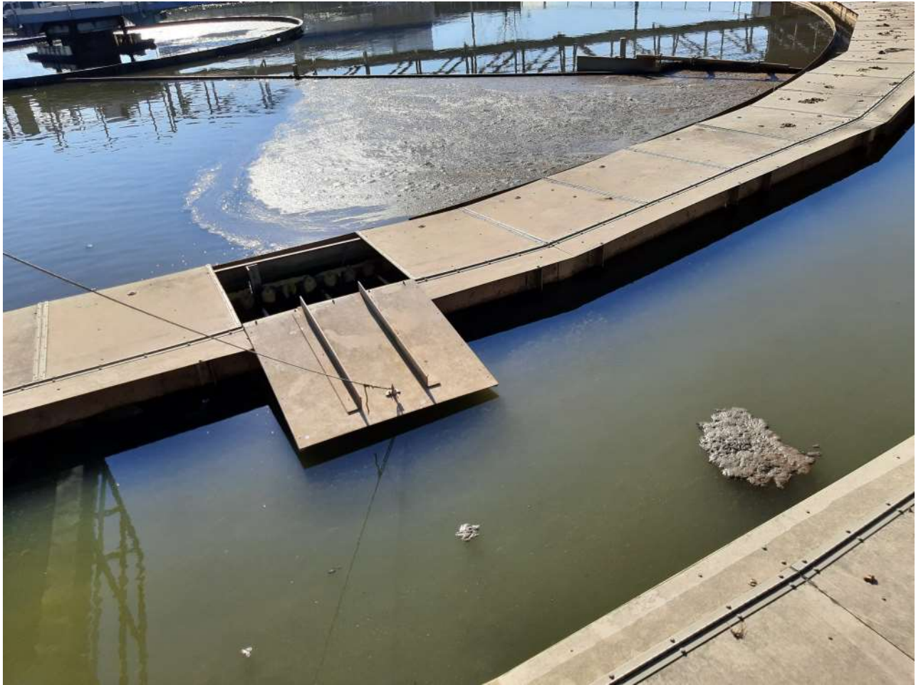
1/30/23 Secondary clarifier #6A scum collection trough/pit was clogged. There was a floating layer of scum on the surface of the water.
