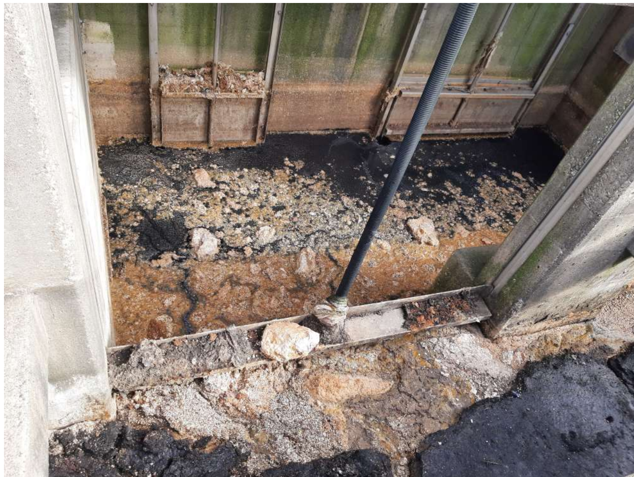
1/30/23 FOG that has breached the PST treatment.
