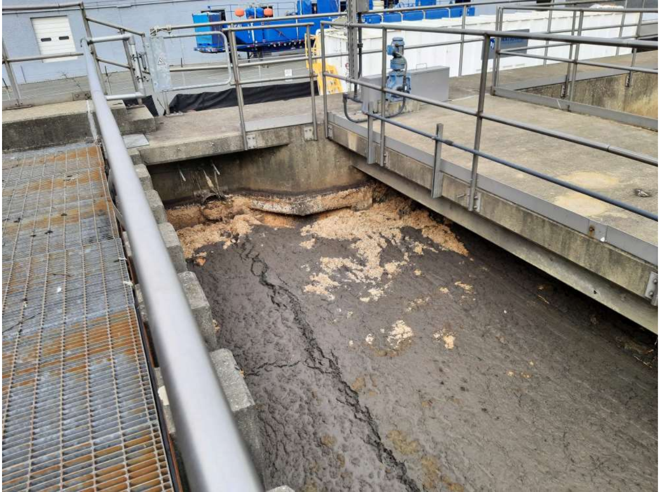
1/30/23 PST #1 has a thick layer of FOG.
