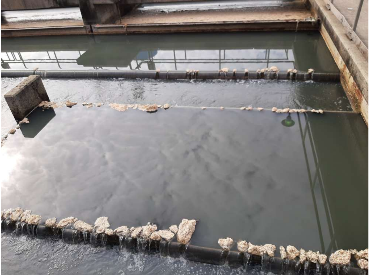
11/30/23 FOG and BAF media clumped together overflowing the PST overflow weirs.
