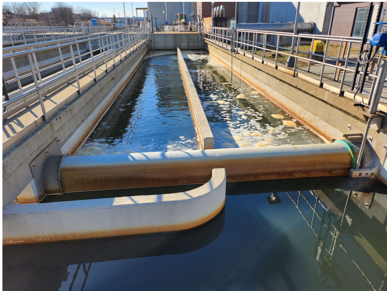
1/30/23 Chlorine contact with scum log
