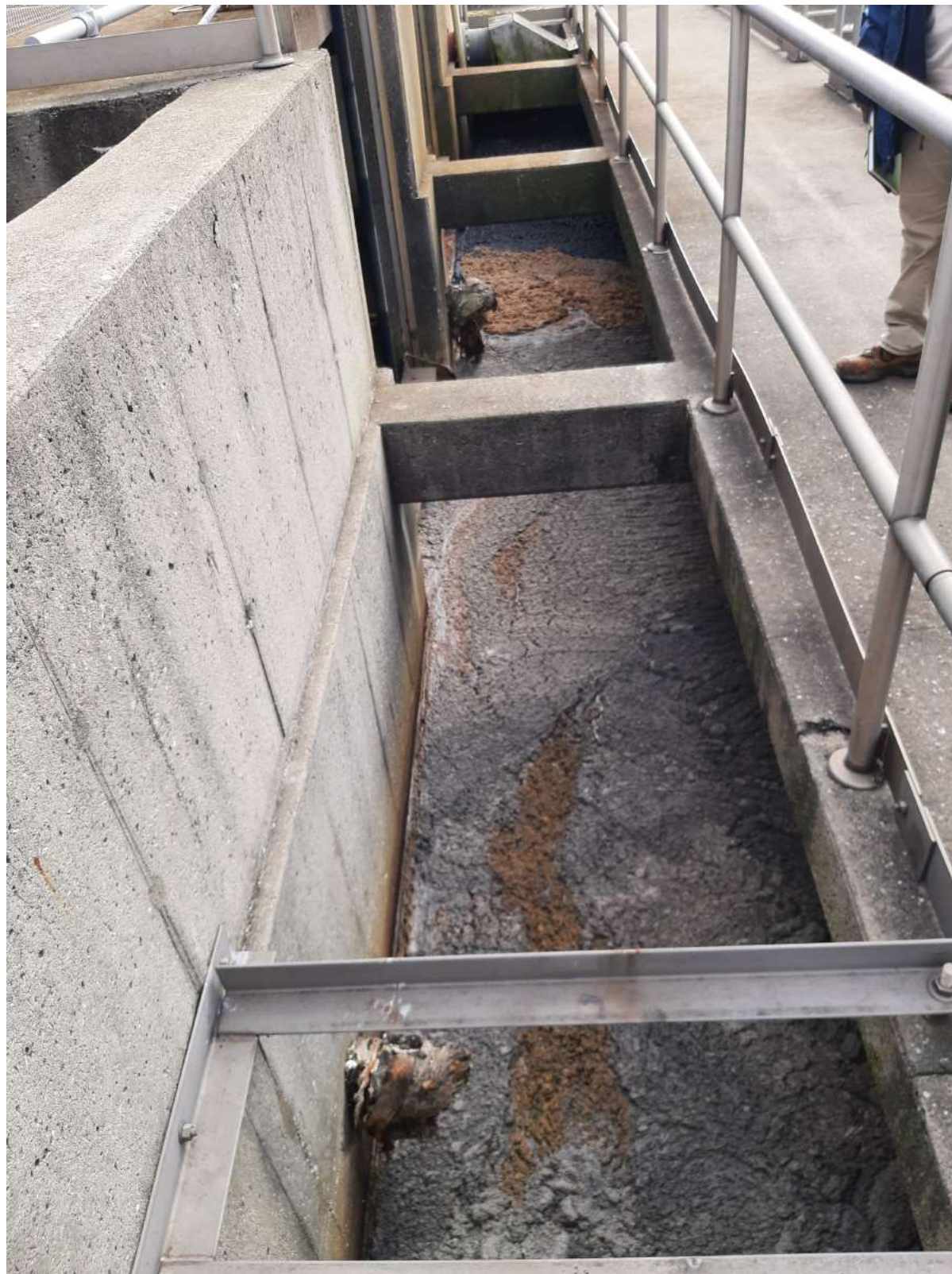
1/30/23 FOG that has breached the weirs of the PSTs.
