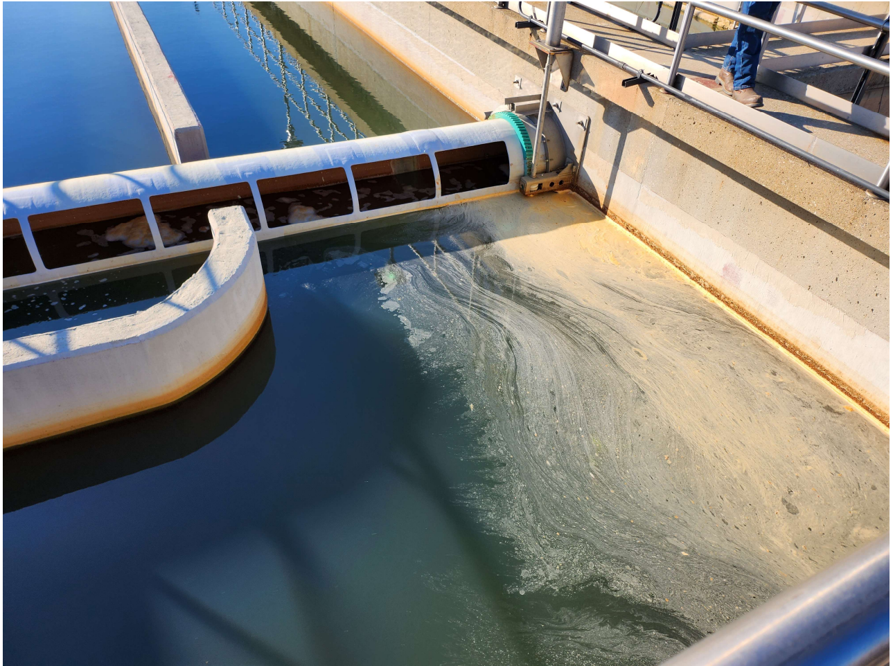
1/30/23 Chlorine contact basin
