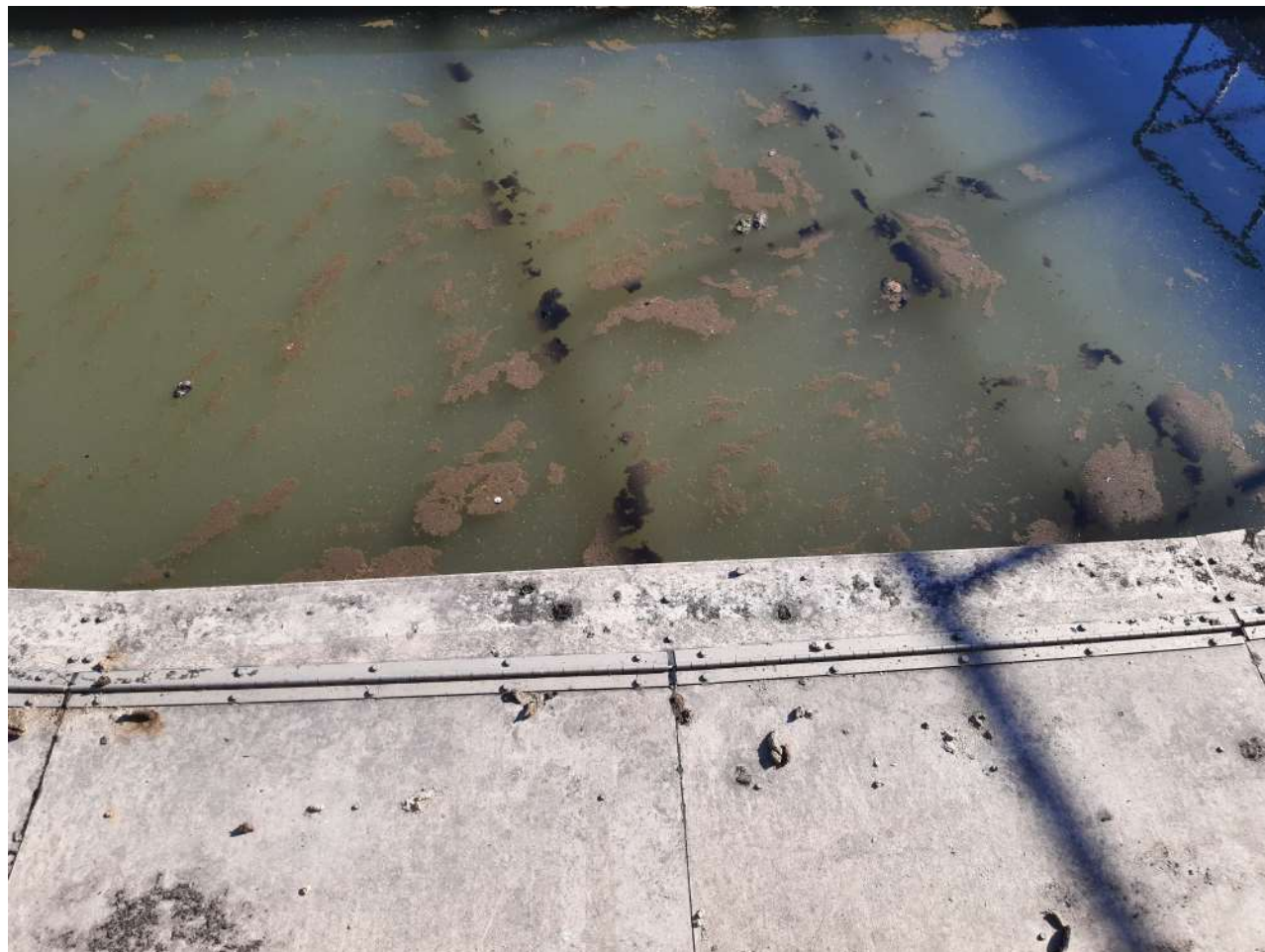
1/30/23 Secondary clarifier 5A with floating biosolids
