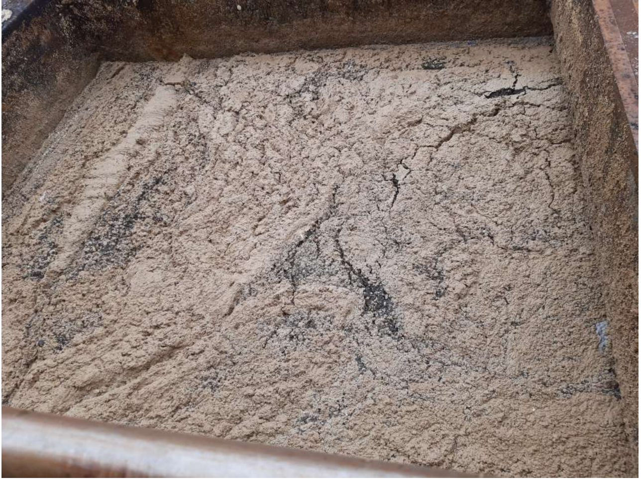
1/30/23 Influent tank at fine screening building showing heavy layer of grease.
