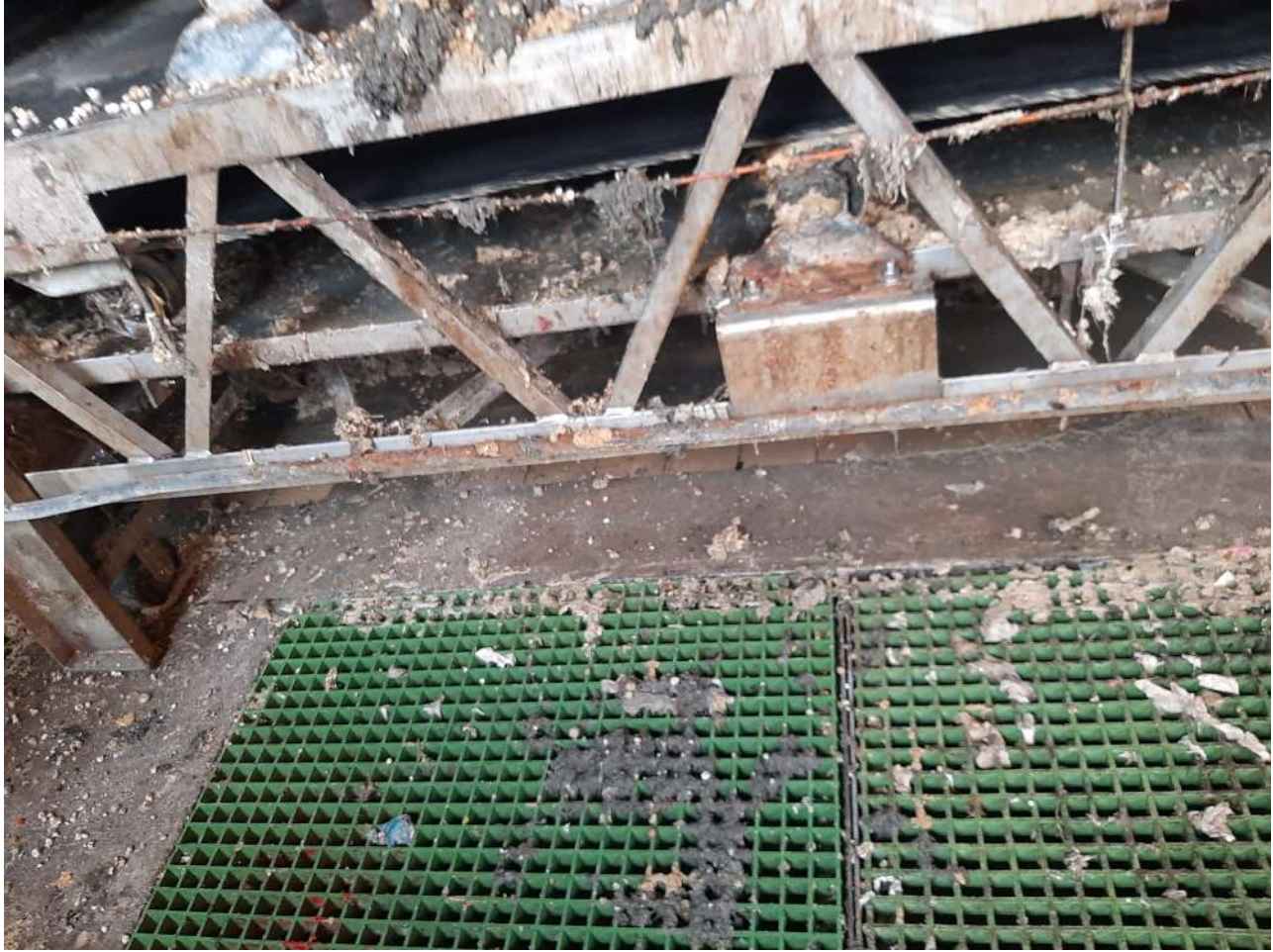
1/30/23 conveyor belt area at fine screening building
