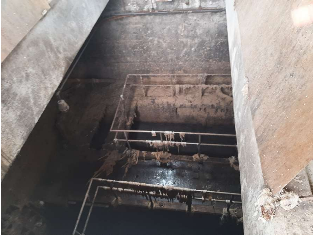
1/30/23 Industrial plant influent. Grease was observed on the screens and floating in the influent.
