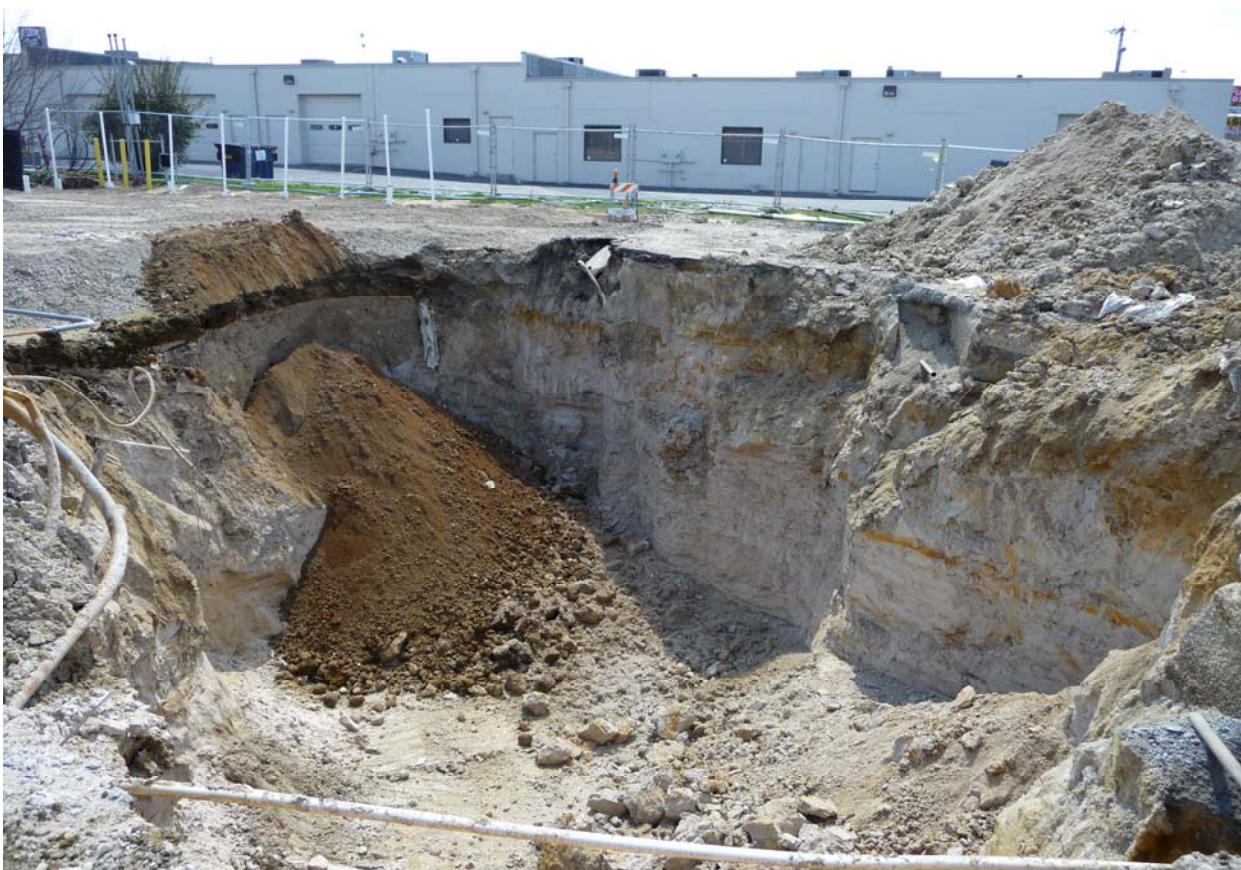
Photo showing over-excavation of the Tank 4 cavity.
