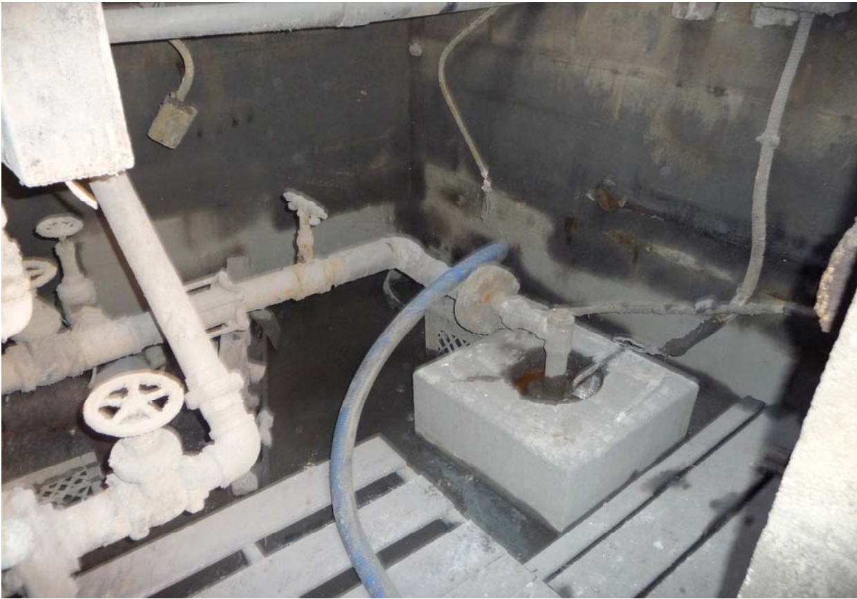
Photo showing the facilities former well house with the well-head featured on the right
