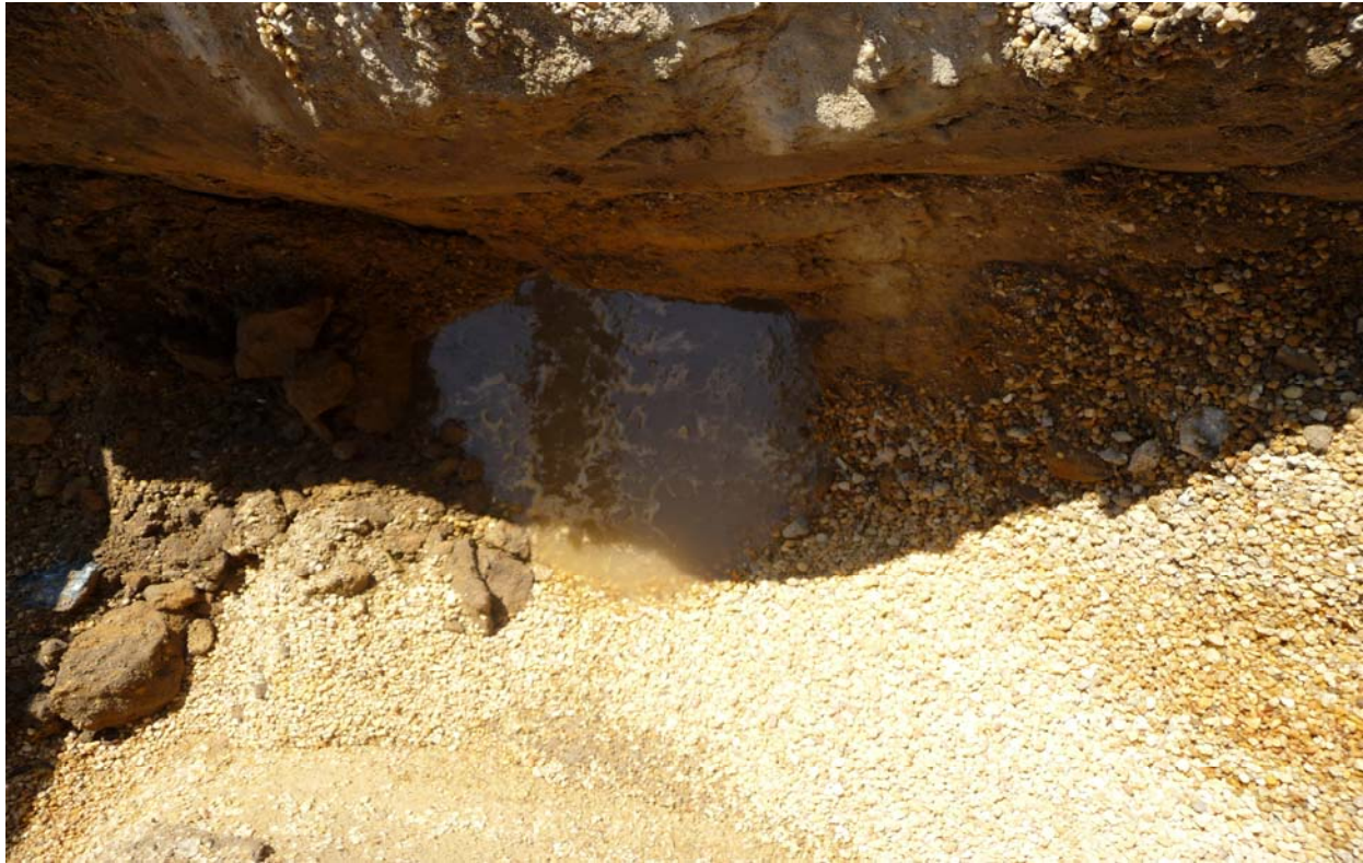
Typical condition of dispenser subgrade showing pea gravel backfill and ponded water.
