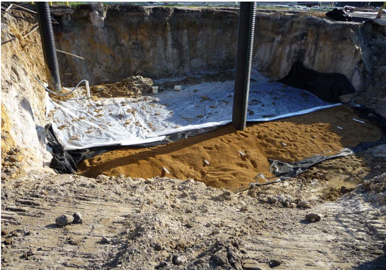
Photo showing a view of remedial piping while under construction. Vertical corrugated pipe were installed as guides for future wells.
