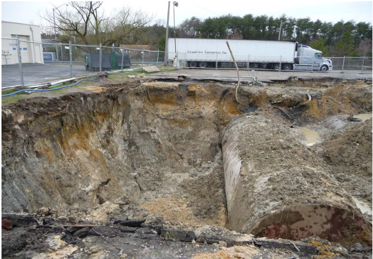
Photo of Tank 3 prior to removal with Tank 2 on right (partially exposed).
