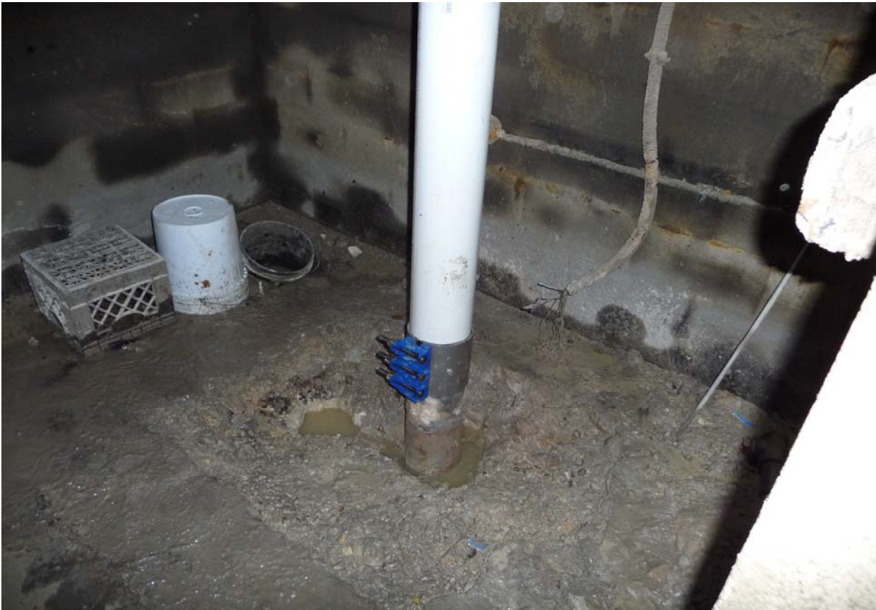
Photo showing the coupling for transition between 6-inch steel casing and 6-inch PVC prior to well-house demolition.
