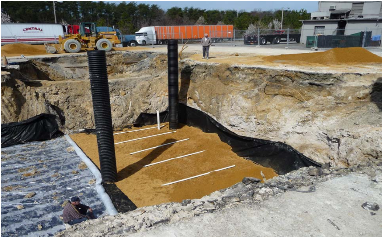
Photo showing a view of remedial piping being installed in the tankfield excavation.
