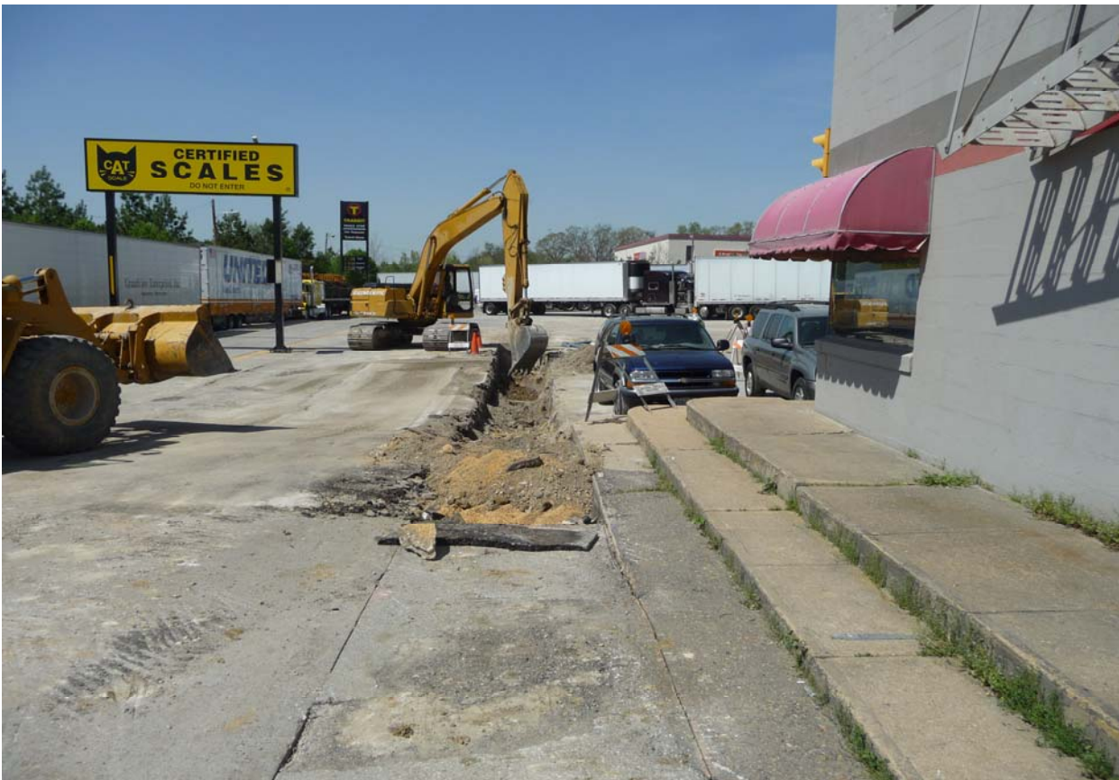
Photo showing excavation of L-Series trench, typical of product pipe excavation and removal.
