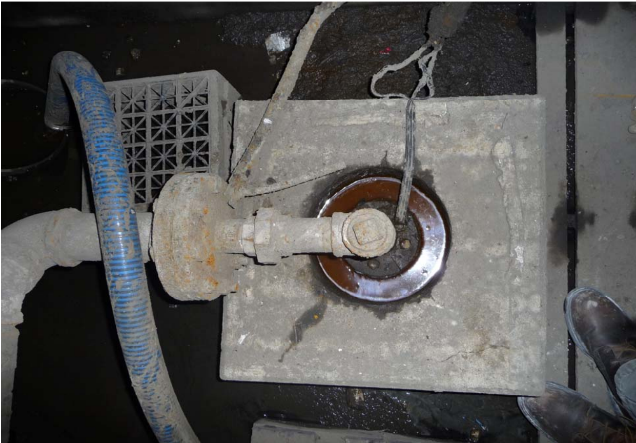
Photo showing the well-head and associated plumbing and electrical supply for the pump
