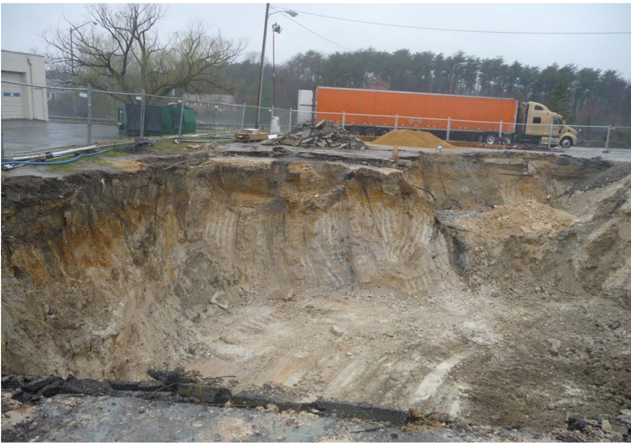
Photo showing over-excavation of the tank cavity for Tanks 1, 2, and 3.
