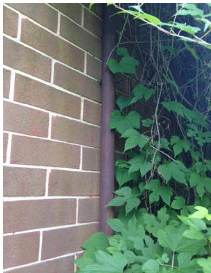
Photo 13: View of existing 10,000-gallon heating oil UST vent piping.
