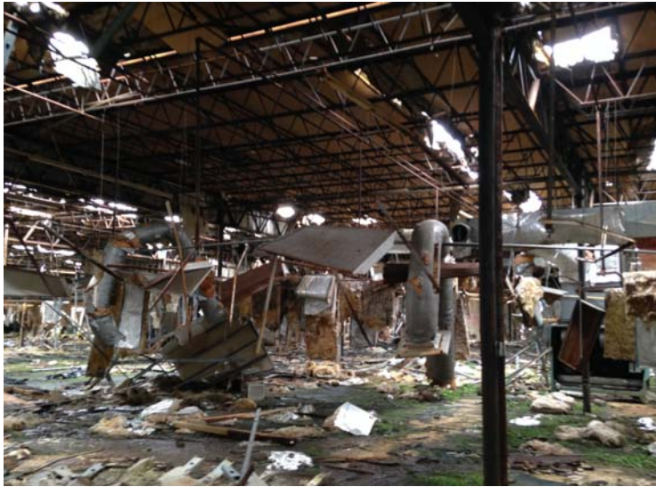
Photo 5: View of interior conditions within vacant warehouse.
