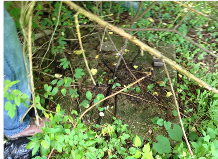
Photo 10: View of suspect fuel dispenser island in the vicinity of the former 10,000-gallon gasoline UST.
