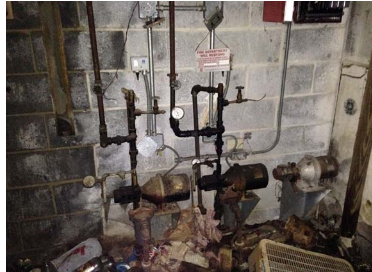
Photo 6: View of transfer pumps associated with the current heating oil UST system.
