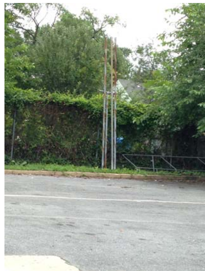
Photo 16: View of vent piping present at 5611 Ager Road.
