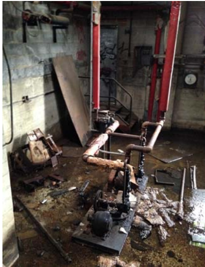
Photo 7: View of piping platform within boiler room.
