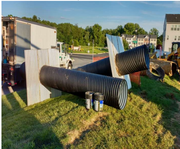
BCCMP Pipe and Uncoated Anti-Seep Collars
