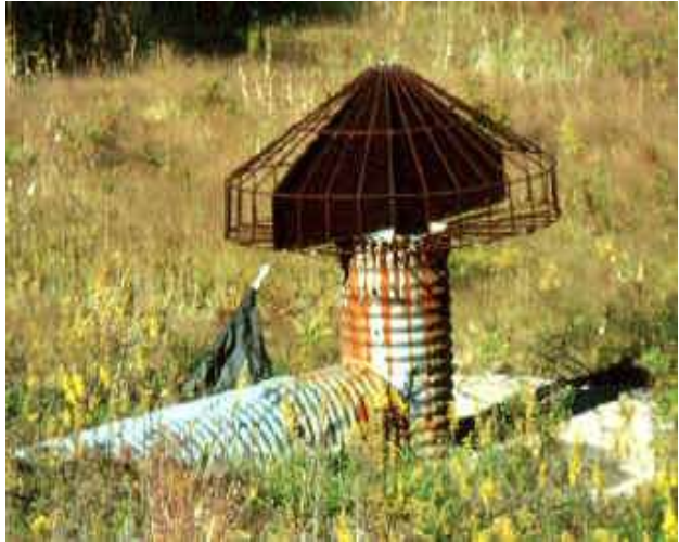
Welded Reinforcing Steel Trash Rack w/Anti-Vortex Baffle (Photo courtesy of HydroCAD Software Solutions, LLC)
