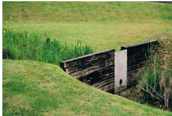
Wooden Weir with Orifice Plate (Photo courtesy of Morton-Roberts Consulting Engineers)
