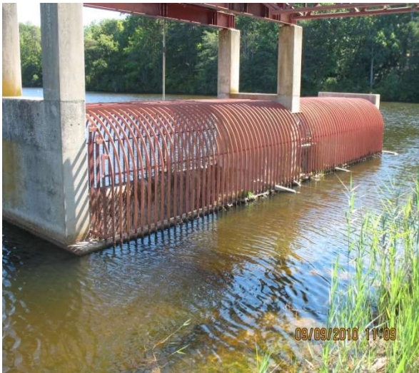
Large Trash Rack on Control Structure (courtesy SWM, LLC.)
