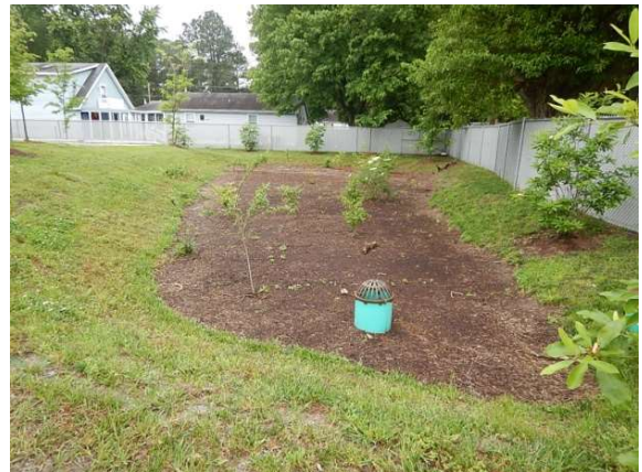
Control Structure in a Micro-Bioretention Filter
