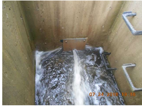
Metal Low-Flow Orifice (Partially Clogged)
