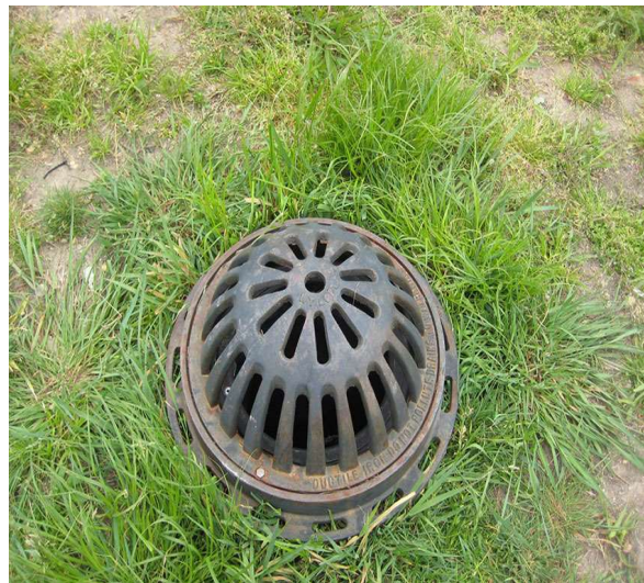
Cast Iron Surface Inlet Trash Rack ("Beehive")
