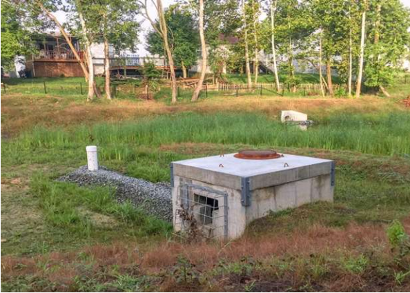
Concrete Control Structure and Low-Flow Dewatering Device (Photo courtesy of Gannett Fleming, Inc.)
