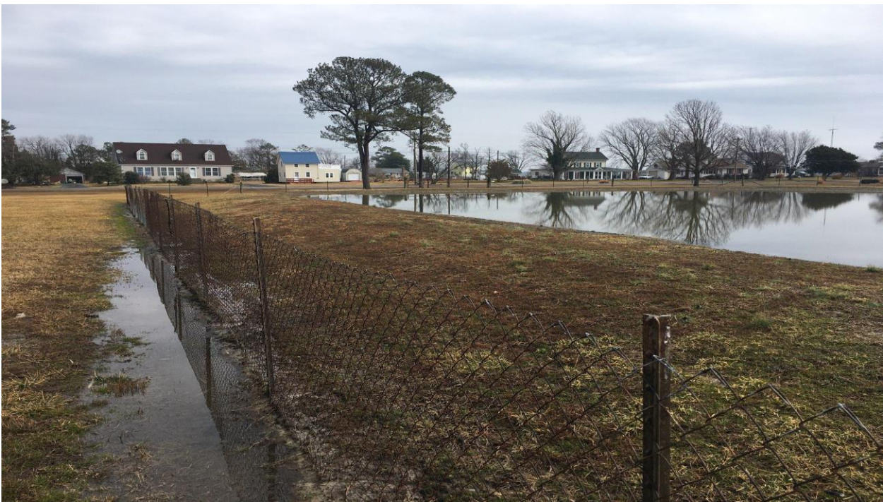
BIP with adequate fencing and vegetation maintenance but has inadequate freeboard (less than 2') and at potential risk of discharge in the event of a storm event.
