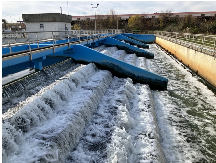
Image 03: Step Aeration system, final effluent.
