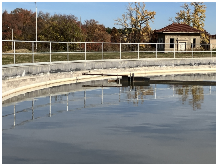
Image 01: PST #11, Missing skimmer flap.
